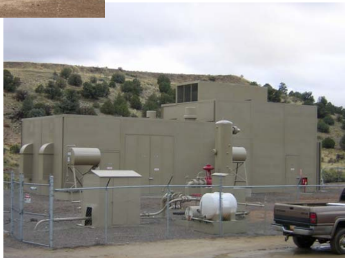
Gas Compressor Sound Enclosure
